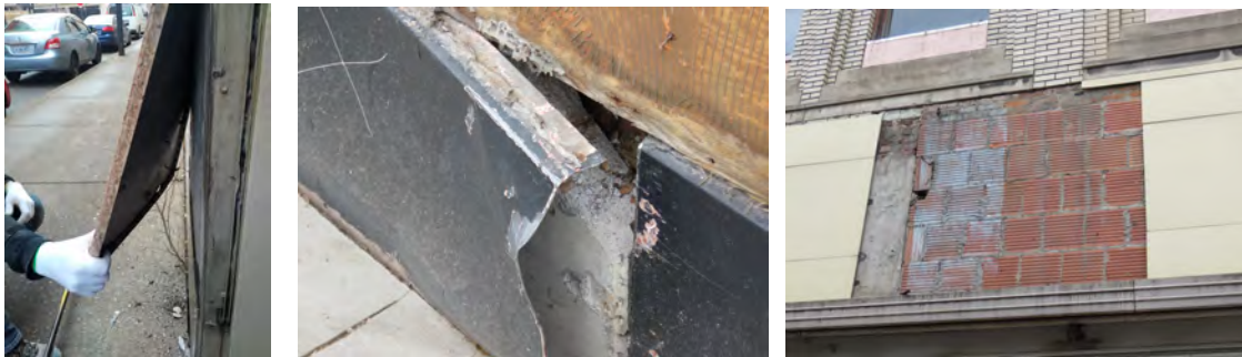
Enameled panels on the King Street elevation painted over with black paint (left and centre) or replaced with synthetic cladding (right).
