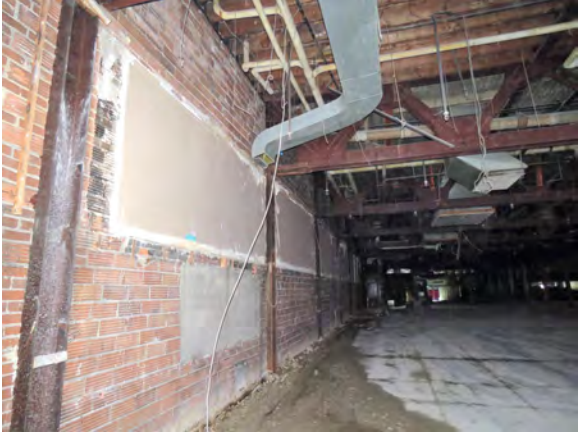
Steel trusses with a 50 foot span supported by steel posts embedded in the exterior masonry wall on Hughson Street.
