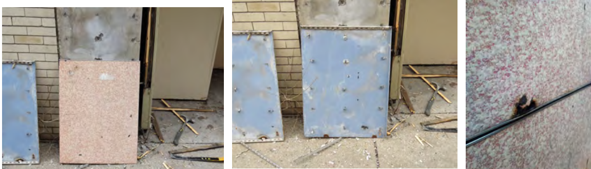
Porcelain enameled panels with concrete backing. Each panel is attached with 15 steel clips. The majority of these clips have corroded through to the surface.
