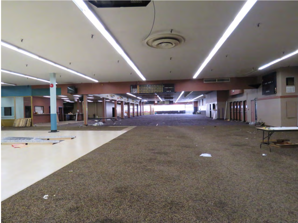
Condition of the ground floor interior just prior to removal of hazardous materials.
