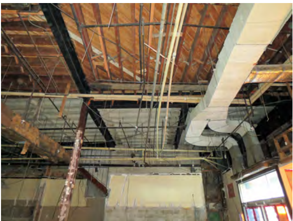
Transition between the wood framing and floors in the older portion of the building and the pre-cast concrete slab floors in the later additions.
