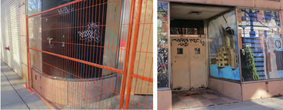
The entrances on King William Street retain some original features but are generally in poor condition.
