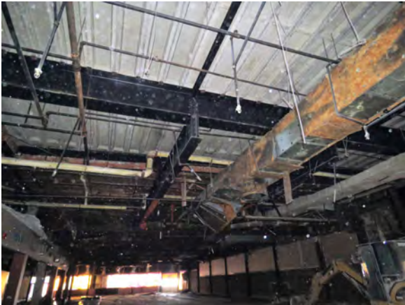
Steel frame and pre-cast concrete slab floor construction in the rear and east portions of the building.
