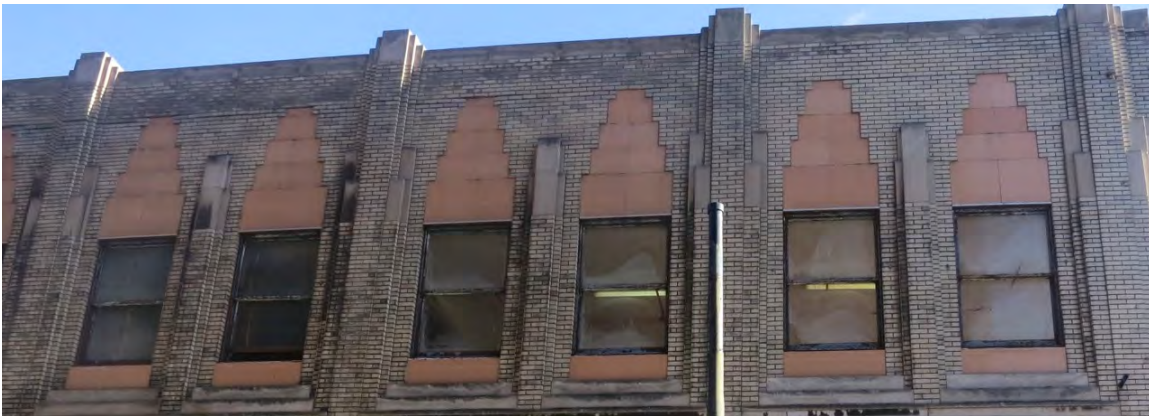
Original steel sash windows on the 2 nd floor are corroded and no longer operable.
