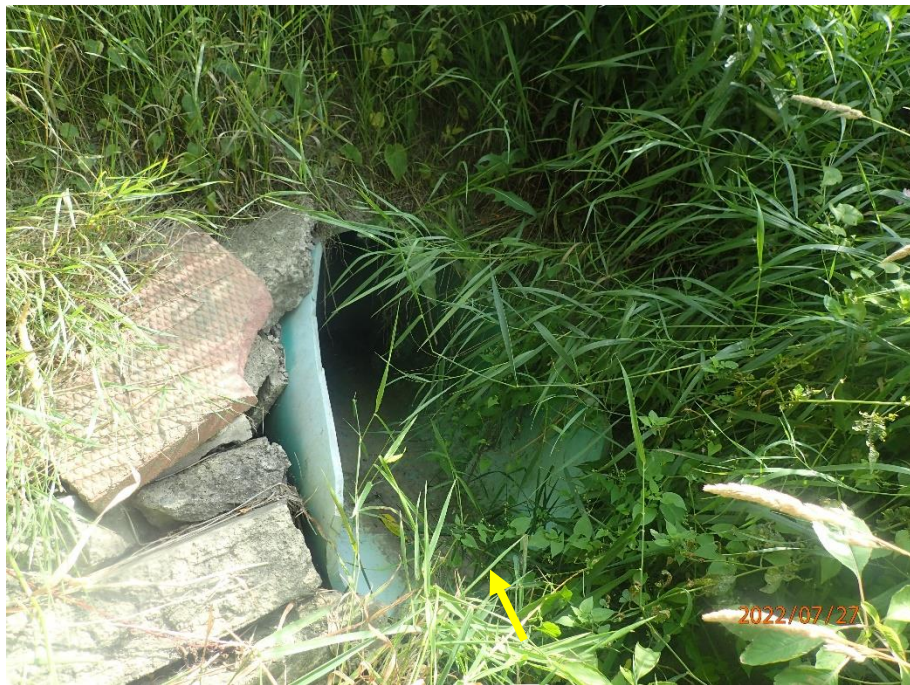
Flows exit the reach through a stable 0.90 m PVC pipe culvert passes beneath Homestead Drive and Upper James Street.
