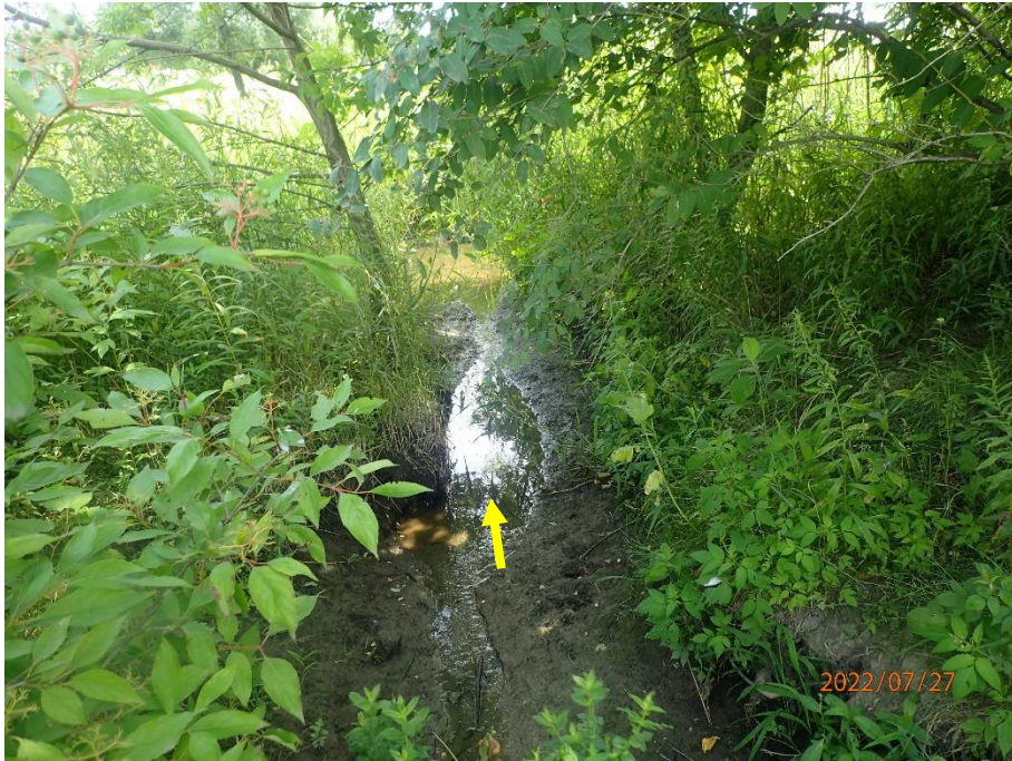
The channel typically exhibits a trapezoidal shape with bank angles generally ranging from 60-90 degrees.
