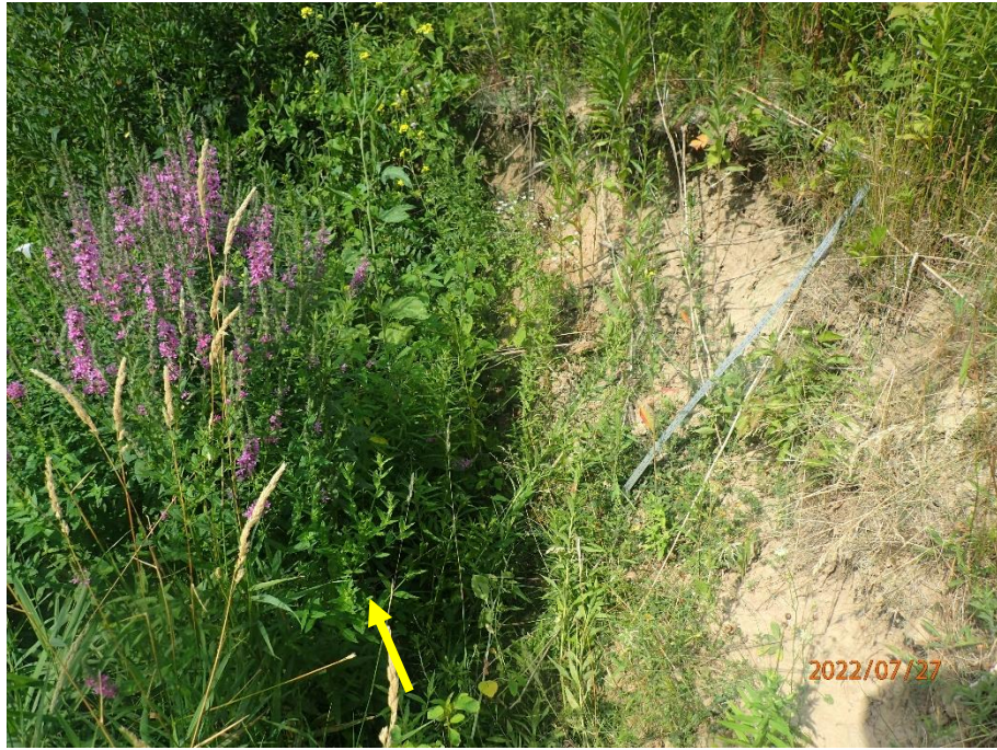
Bank erosion has caused several outer banks to become fully exposed and void of any significant vegetation establishment.
