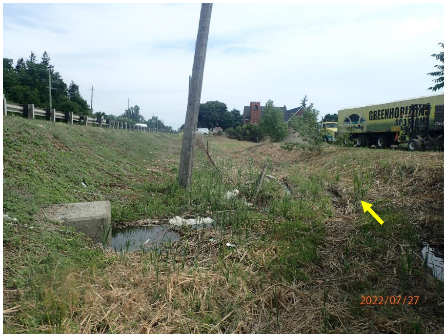
Sections of the reach exhibit multiple and poorly defined channels and flow-paths.
