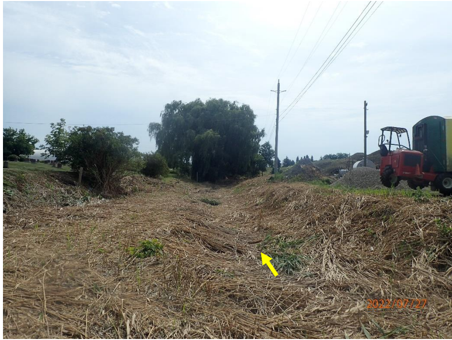
Cattail vegetation encroachment is significant throughout the downstream portions of the reach. The channel here is poorly defined.
