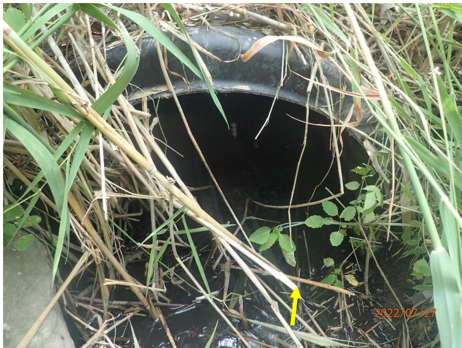
Flows exit reach H1S2 through a stable corrugated plastic pipe culvert that passes beneath a service road associated with the adjacent sod farm.
