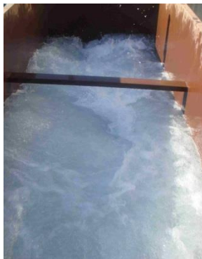
Inside View of Hopper Agitator
