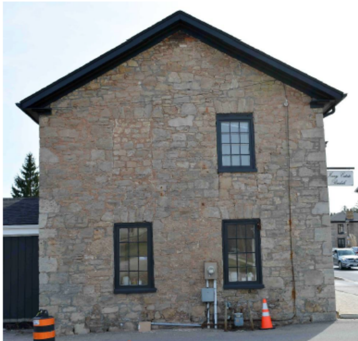
Figure 5: North Wall Damage
