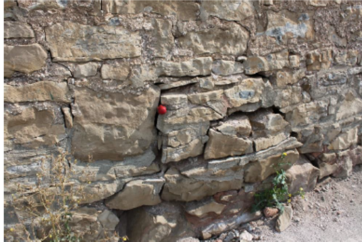
Figure 4: South Wall Damage
