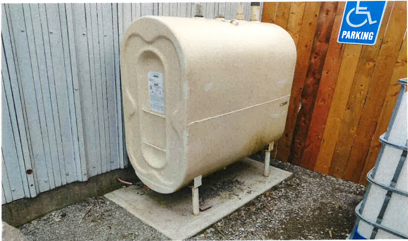
View of fuel oil AST to the west of the barn in the north-western portion of the subject site (looking south)
