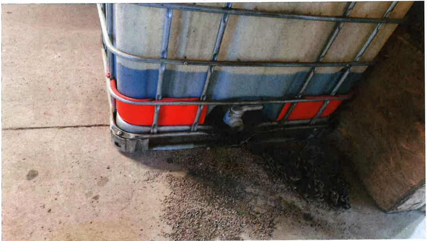
View of waste oil AST inside the northern barn in the north-eastern portion of the subject site
