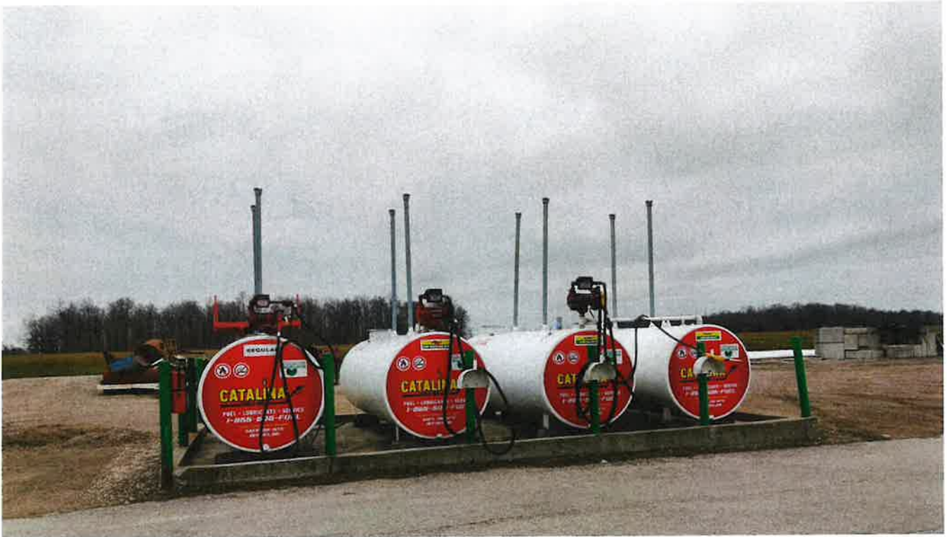
View of four (4) fuel oil ASTs located in the north-eastern portion of the subject site (looking south)
