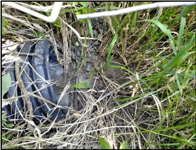
Photograph 49. Upstream View of No Flow Entering Culvert Associated with DF18a Taken in Round 3. View: N Date Taken: July 8, 2024 Site: Parcel 2
